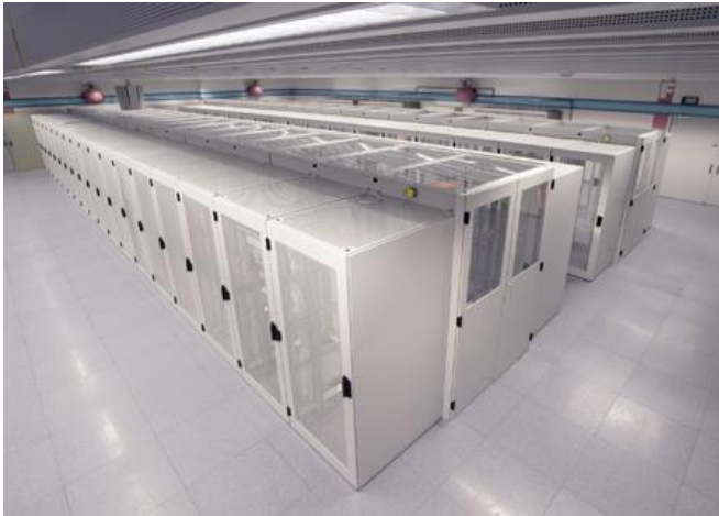
Cold Isle Containment in New Datacenter
