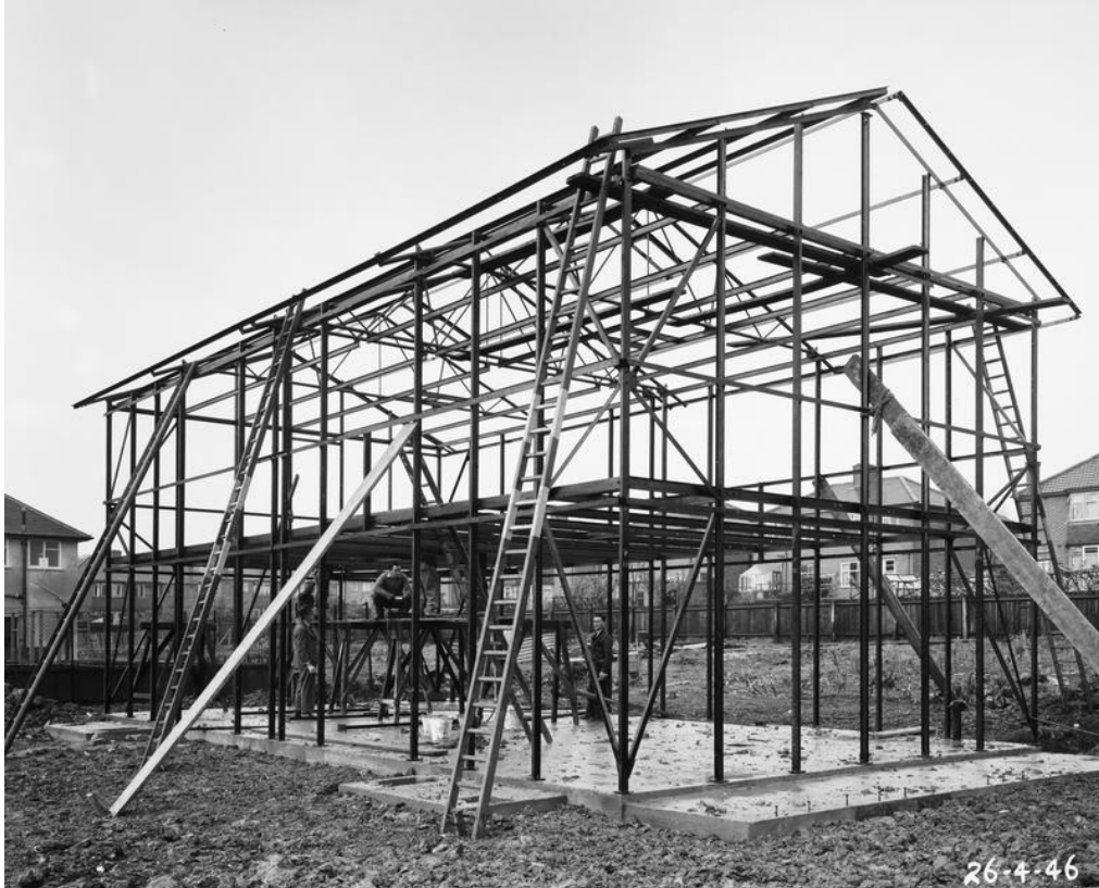
Steel frame BISF house under construction in 1946. Source: Historic England Archive/John Laing Photographic Collection/PA
