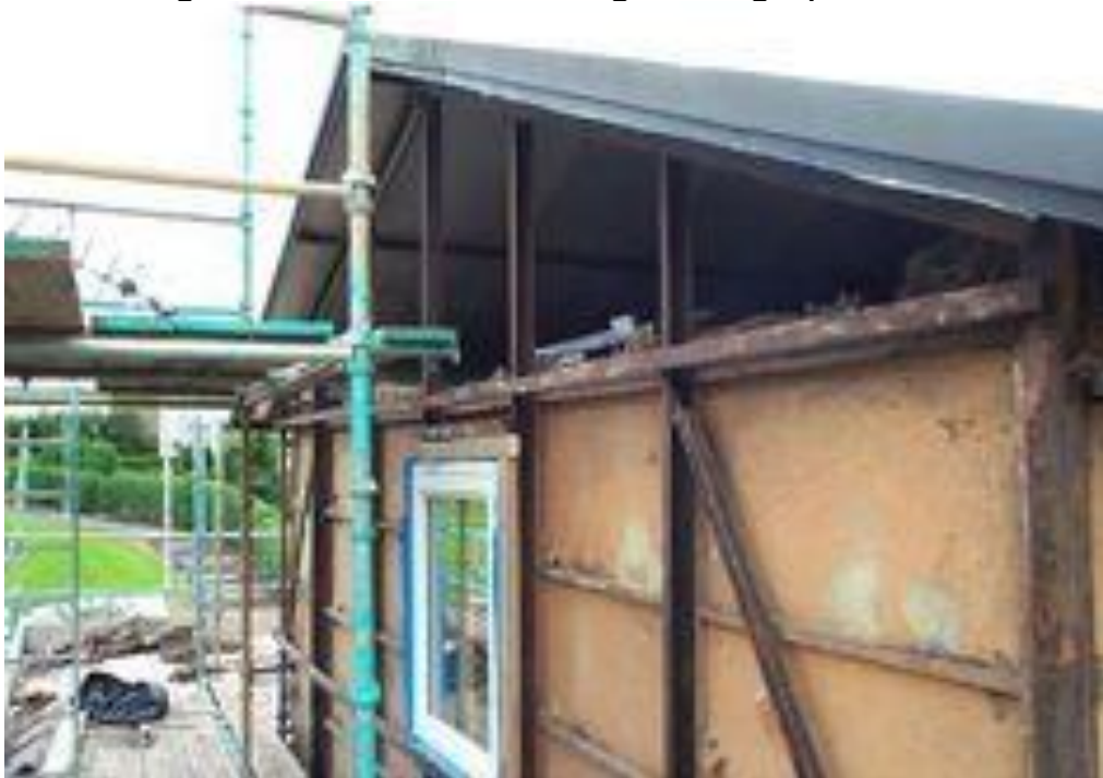
Close-up of steel frame structure of a BISF house during renovation. Source: https://www.pinterest.co.uk/pin/832532681090205638/
