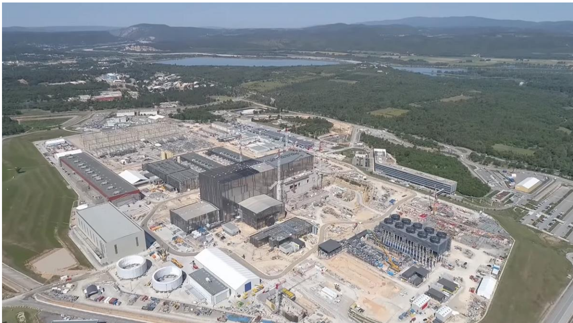
The ITER site in 2020, being built next to the Cadarache facility in Saint-Paul-lès-Durance, in Provence, southern France.
