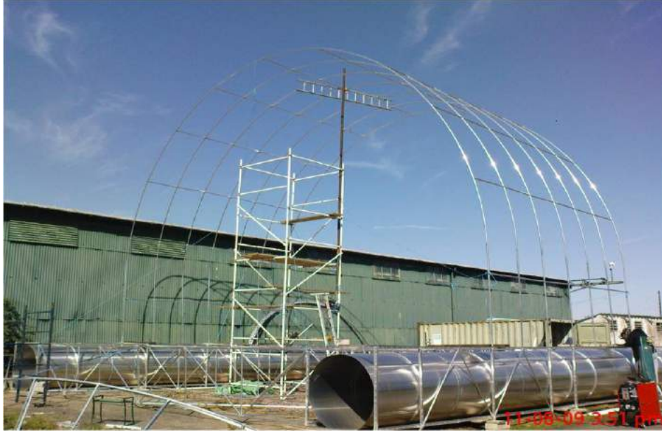
Start of the tubular framework for one variable lift unit showing the positions of the two receiver tanks. Source: Varialift.
