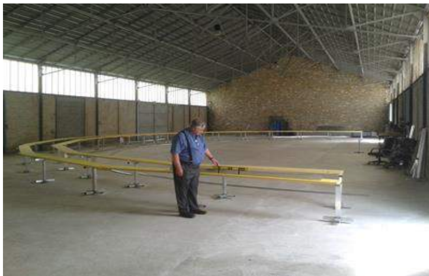
Wooden "jig" on which the semicircular hull frames are built. The frames measure 40 m (131 ft) along the curve; 25 m (82 ft) in diameter. Source: Varialift.
