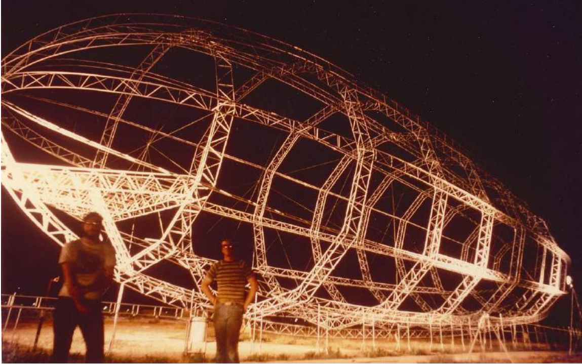
The Conrad CA220 dirigible hull under construction at night. Source: Darwin Conrad via MakeHigleyHistoric
