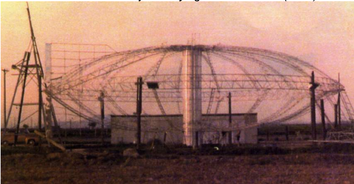
Profile view of the CA80 lenticular airship hull under construction. Note the dorsal and ventral fin structure, left. Source: Darwin Conrad via MakeHigleyHistoric
