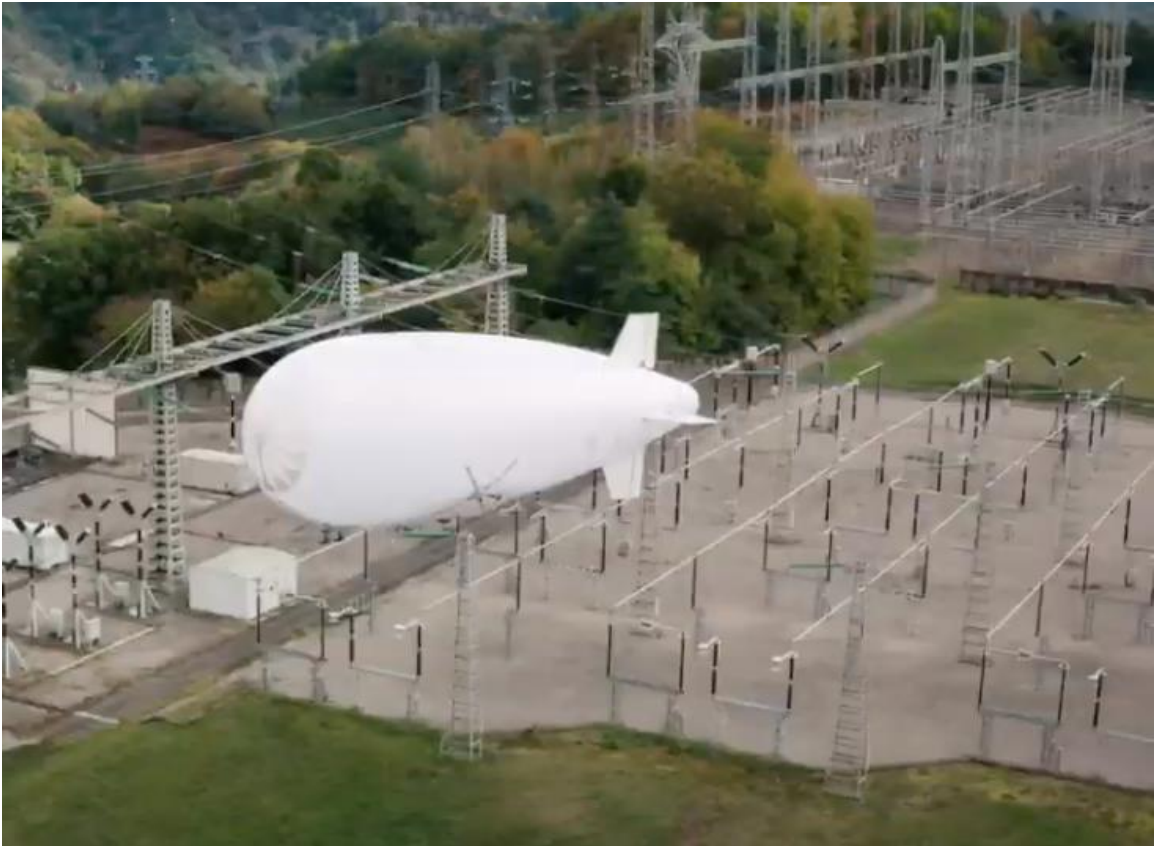
Diridrone flying over an RTE switchyard. Source: Screenshot from RTE video (Dec 2020)
